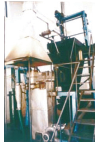
The biomass gasifier is the main source of power during the day
