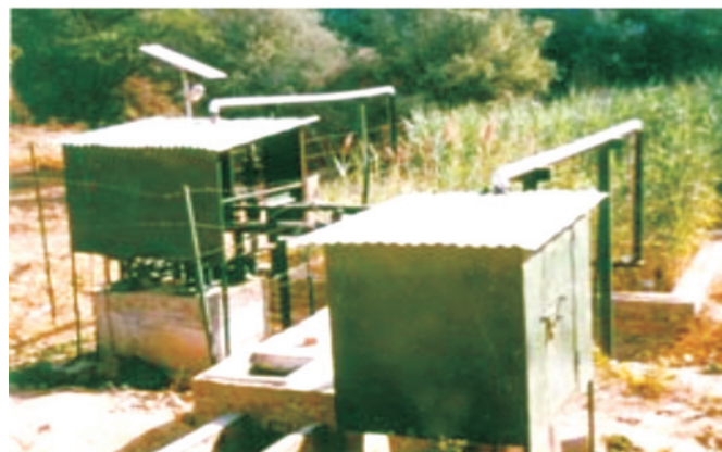
Waste water is recycled by the 'root zone' technique, in which the roots of plants with special capabilities are used to clean the water which is used for irrigation purposes
