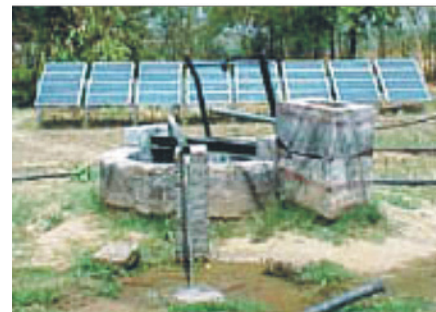
PV-based water pump
