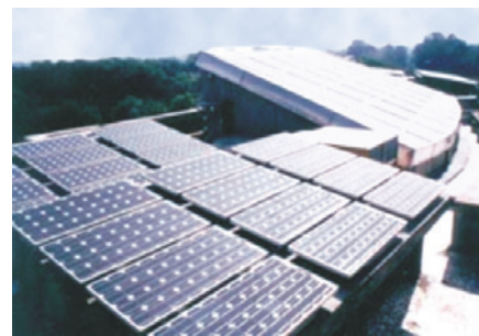
Photovoltaic panels cover the entire roof
