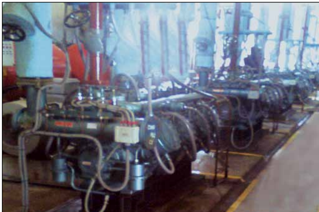
Figure 4 : Bank of four KC93 Kirloskar two-stage compressors.
