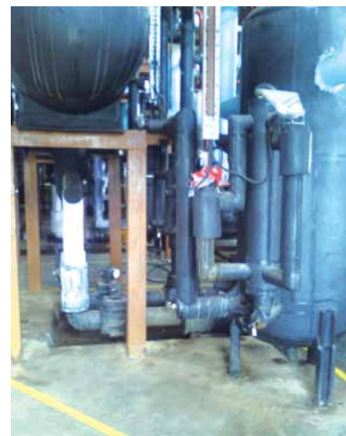
Figure 12 : Ammonia pumps in operation
