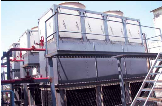
Figure 6 : Evapco make evaporative condensers
