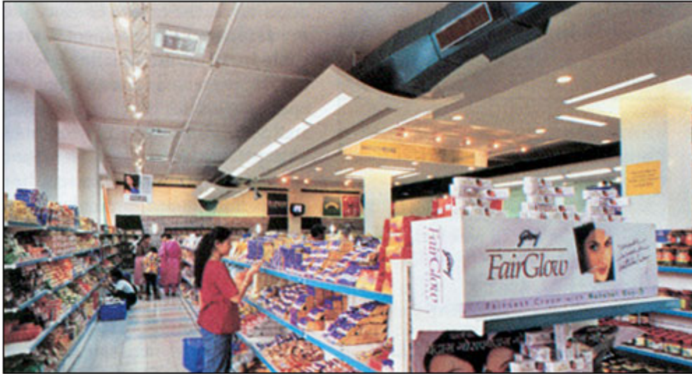
Exposed ducting in a shopping centre. Photo courtesy of Haiko Shopping Centre, Powai, Mumbai
