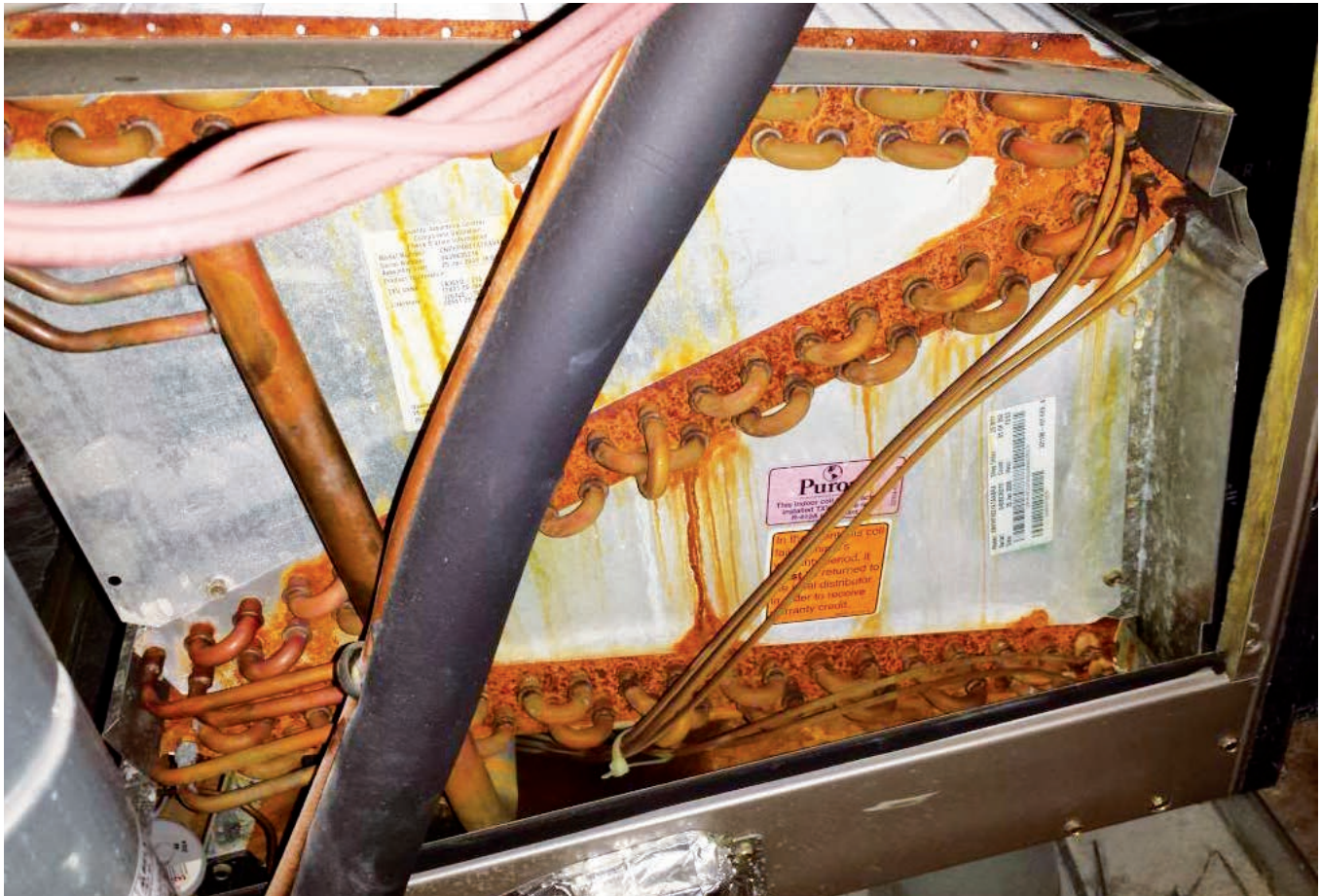
Formic acid corrosion in a coil
