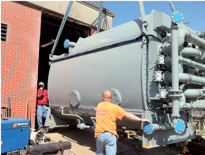
Figure 8: A 150-ton adsorption chiller being installed in the USA
