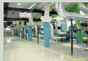
Chillers at Indira Gandhi (IG) Sports Complex
