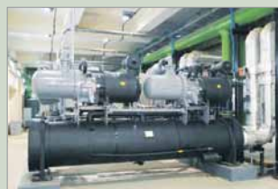
Chillers at Jawaharlal Nehru Stadium
