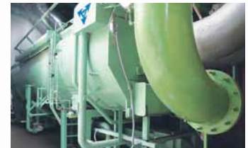
Absorption Chiller fired by exhaust from gas turbine
