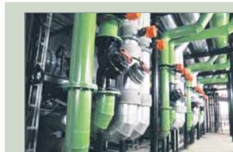
Chilled water piping at Thyagaraj Stadium
