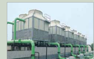
Cooling towers at IG Sports Complex, Delhi's 2nd-largest HVAC installation
