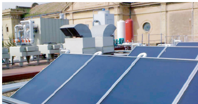
Photo 2: Comfort cooling through a single effect solar absorption machine in Spain
