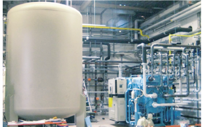
Photo 3: A single-double effect absorption chiller installation in Germany
