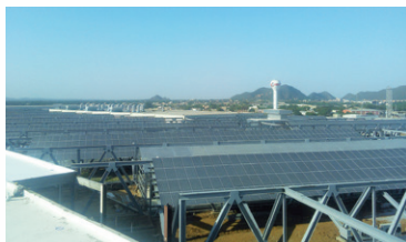
On-site solar photovoltaic cells
