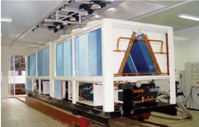
Figure 6 : An air cooled brine chiller.
