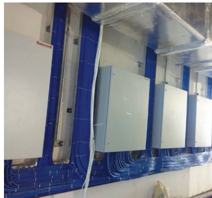
Photo 2: Cables routed neatly and wrapped with tie
