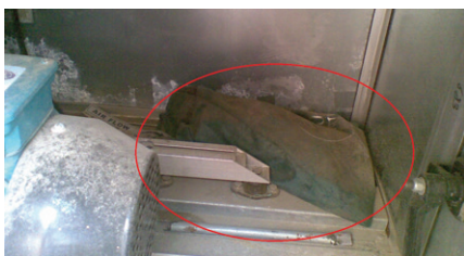
Photo 9: Debris inside AHU
