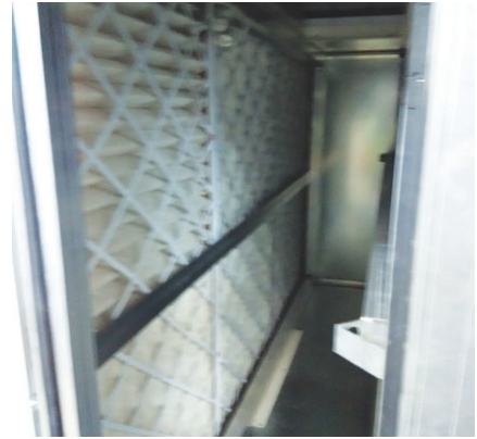
Photo 3: Commissioning filters used during AHU commissioning
