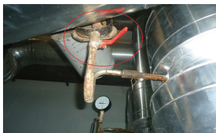
Photo 13: Gauge installed at location that is not visible
