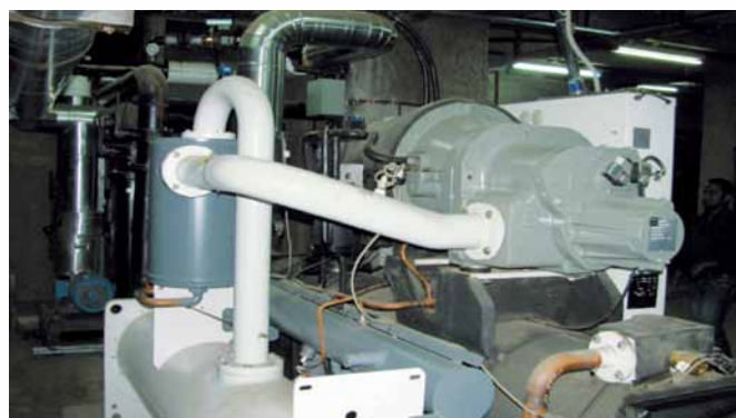
Photo 3: New screw chiller that replaced the old condensing unit
