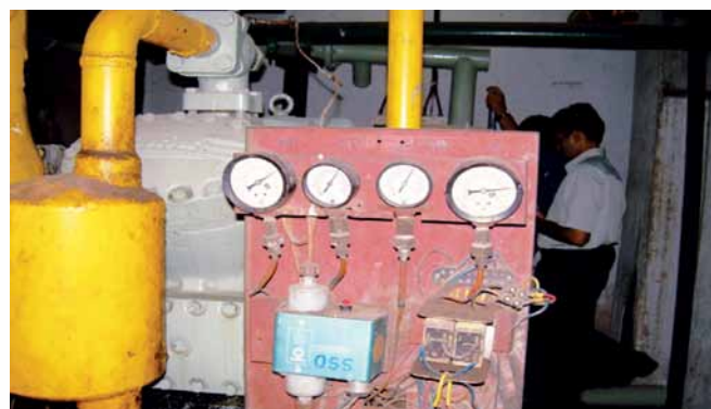
Photo 2: Old reciprocating condensing unit
