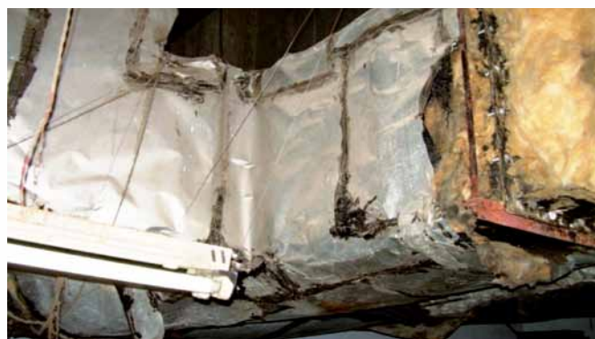
Photo 1: Old main duct from AHU
