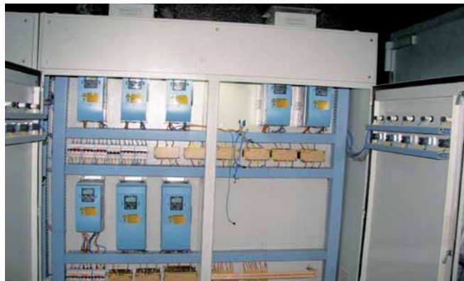
Photo 6: New HVAC panel that houses VFDs and digital energy meters
