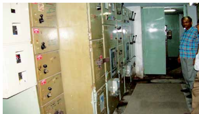
Photo 4: Old HT panels
