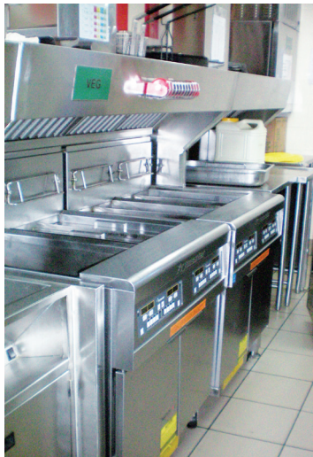
Vats in a kitchen with hood
