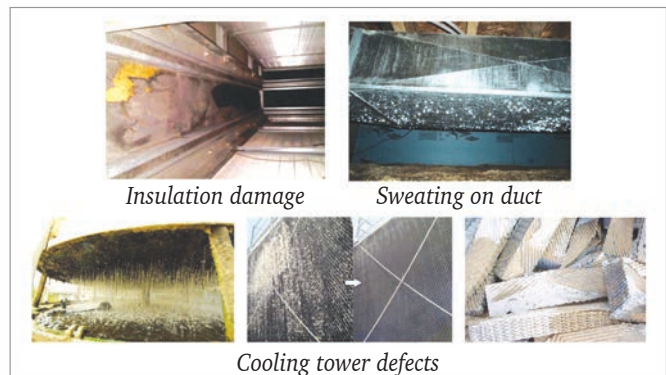
Figure 28: Typical defects found during inspection
