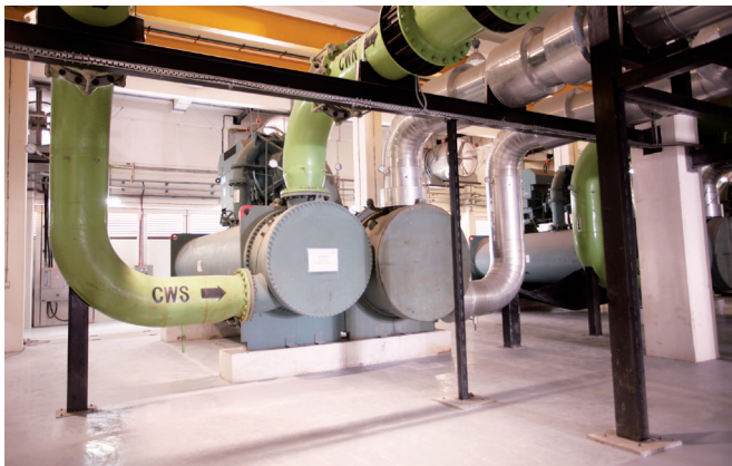
Photo 1: 2500TR centrifugal chillers with interconnecting piping
