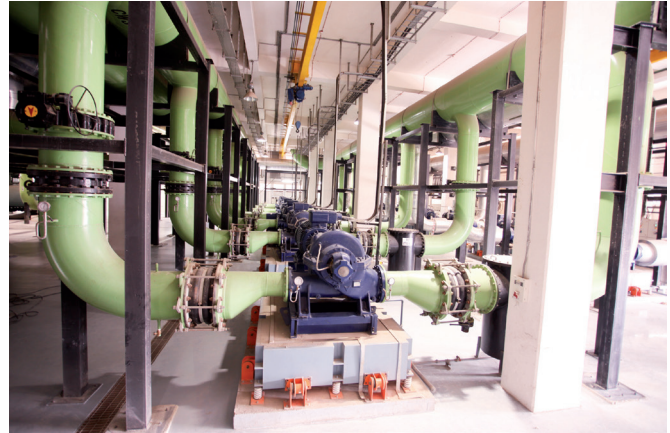
Photo 6: Condenser water pumps with 1300mm headers
