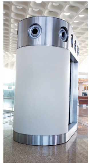
Photo 8: An air tower with jet nozzle outlets in the security hold area
