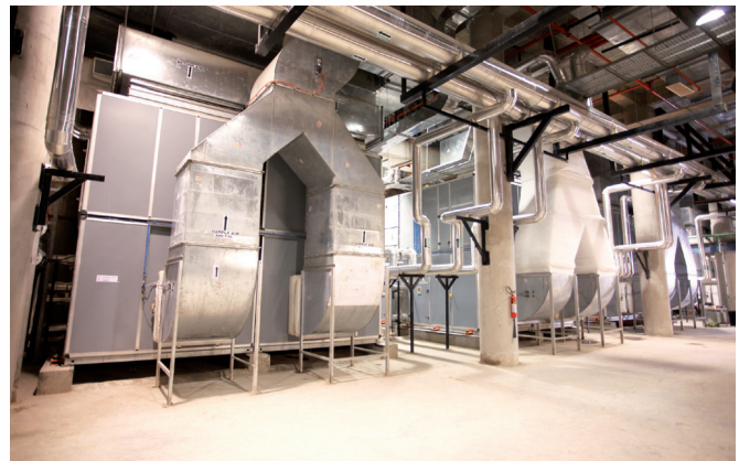
Photo 2: AHU duct and pipe connections
