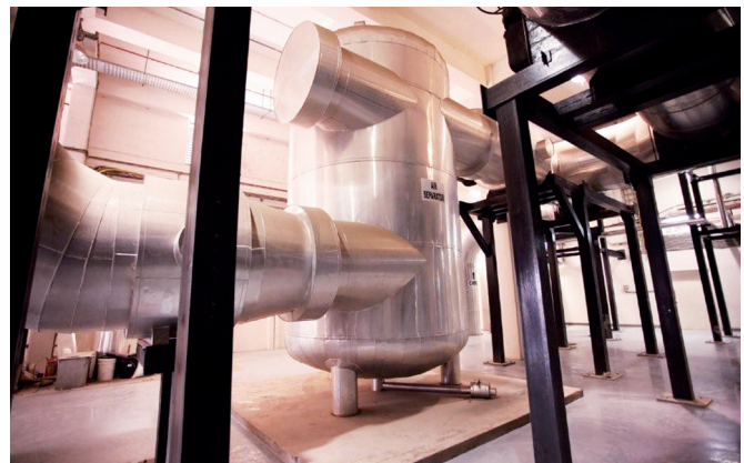
Photo 4: Air separator with 1100mm dia chilled water main header
