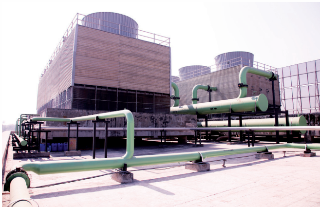
Photo 7: Cooling tower cells 2500TRx6
