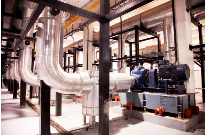
Photo 5: Chilled water pumps with 1100mm headers
