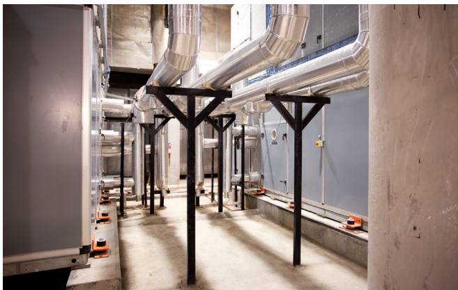
Photo 3: AHU pipe connections with supports
