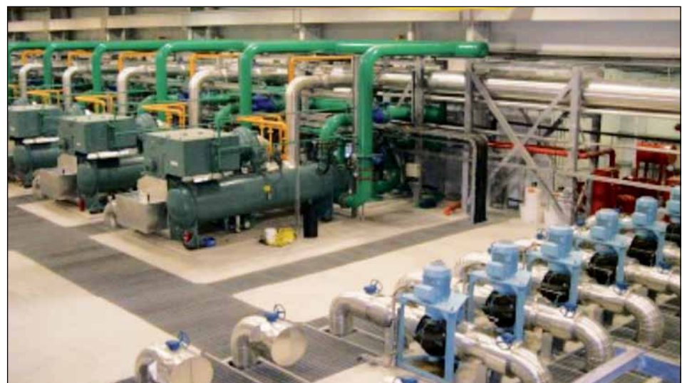
Photo 2: A typical District Cooling centre
