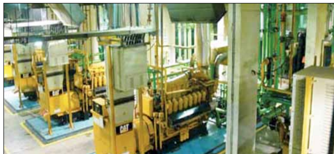
Photo 3: 10MWe BCHP plant at DLF
