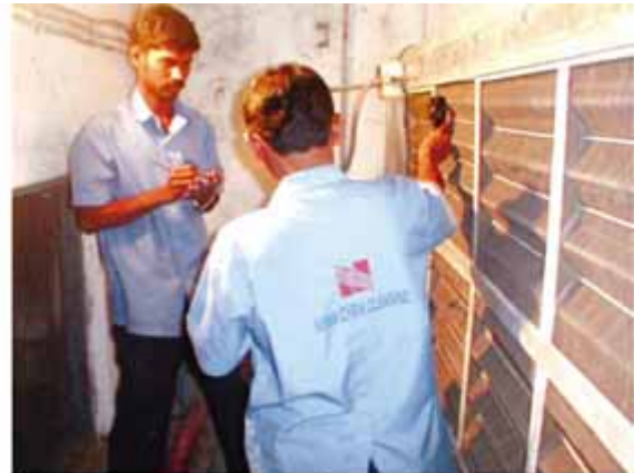
Air quantity recorded with filter after cleaning the coil.
