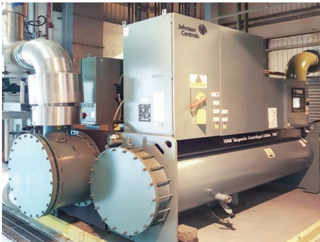
Figure 6: A magnetic bearing chiller installation
