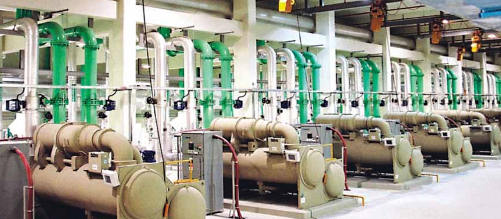
A typical district cooling plant room
