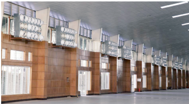
21 diffusers at the end of each plenum
