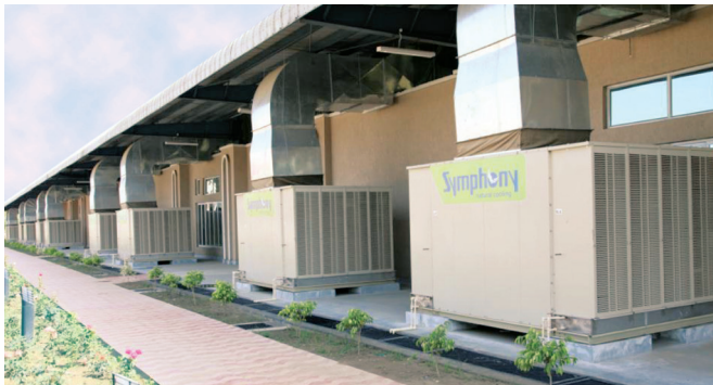
Eleven evaporative coolers are installed on each side of the hall
