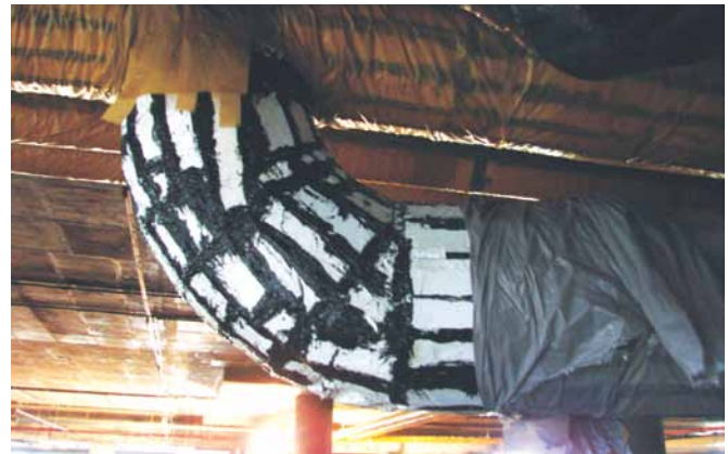
Photo 5 : Multiple joints in the insulation for large diameter pipes.
