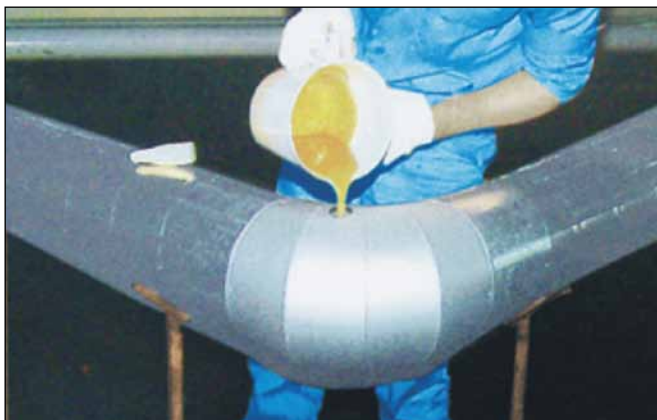
Photo 8 : A standard fabricated outer casing is placed over the elbow and filled with PUF chemicals.
