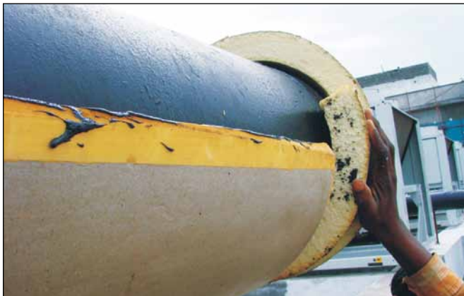
Photo 3 : Air gap between pipe & insulation for field applied insulation.
