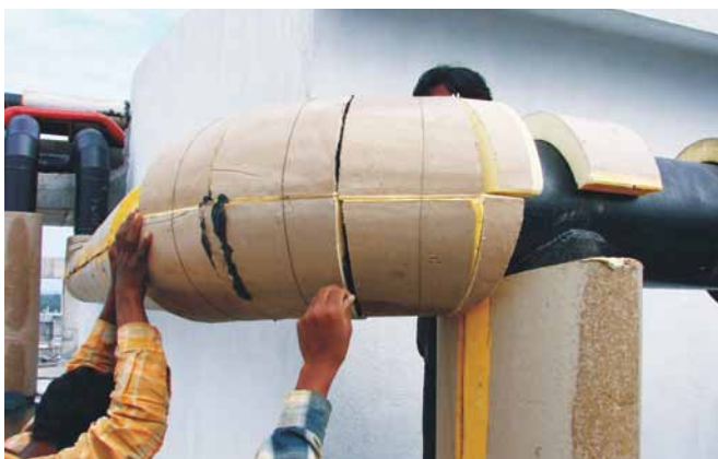
Photo 4 : Insulation joints not staggered have large gaps in circumferential joints.
