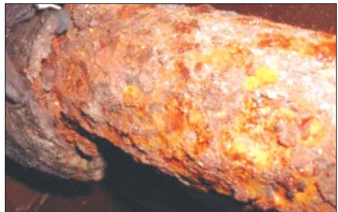
Photo 9 : Corrosion in supply chilled water pipe pipe
