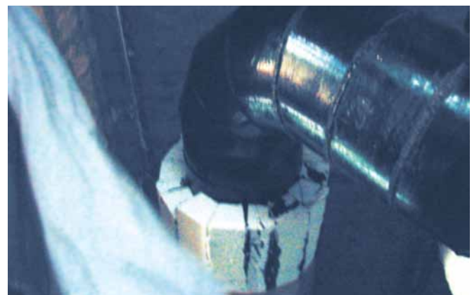
Photo 6 : Large diameter pipe insulation using trapezoidal insulation sections. Notice the gaps between longitudinal sections and between insulation and pipe.
