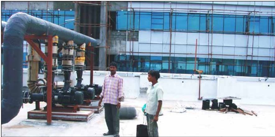
Photo 1 : Typical scene at a site where insulation work is being done. Notice the open flame for melting the bitumen and then hand carrying it to where needed for sticking the insulation to the pipe.
