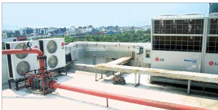
VRF and split units installed on the school terrace
