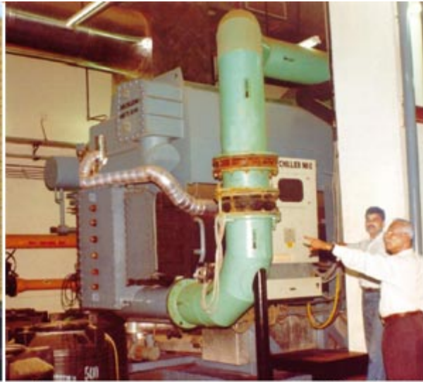
Absorption chiller in the plant room of Grand Hyatt Mumbai. Photo courtesy of Grand Hyatt Mumbai.
