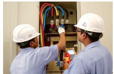
Figure 16: Measurement of electrical parameters on HVAC rotary equipment MCC
