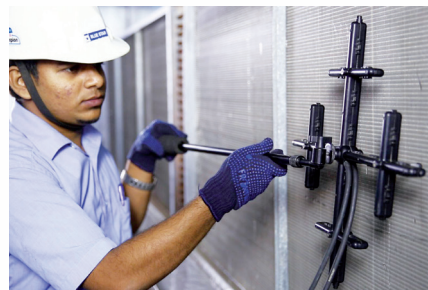
Figure 15: Air velocity measurement on a cooling coil with an air matrix station comprising 16 pitot tube manometers in a 50000cfm floor mounted AHU
