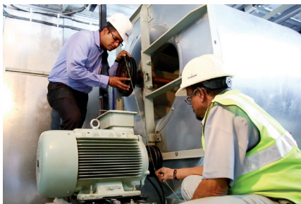
Figure 14: Alignment of a 25000cfm fan with motor inside a floor mounted double skin AHU, housing two such fans
