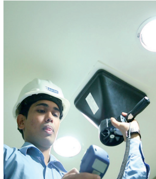
Figure 8: Air volume hood
