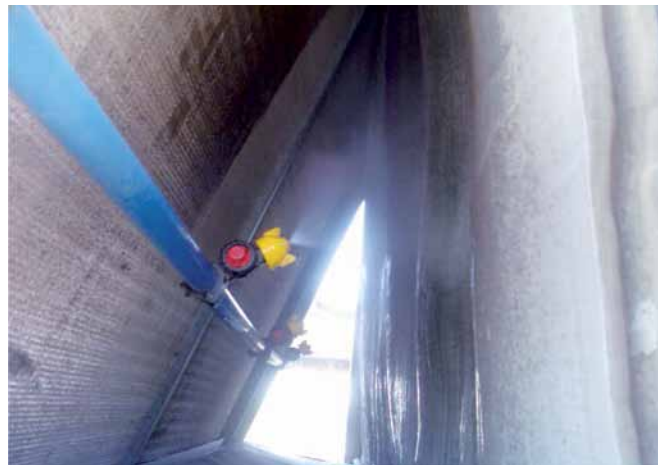
Photo 2 : Sensible air pre-cooling system in operation
