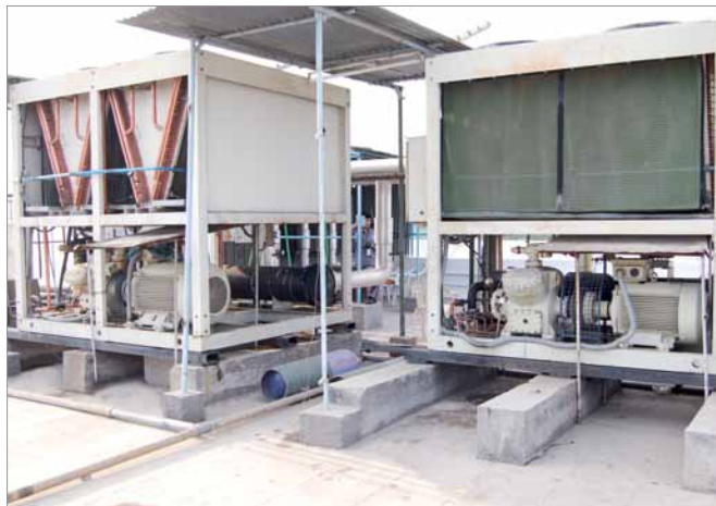
Photo 1 : Air-cooled chillers with sensible air pre-cooling system and shades
