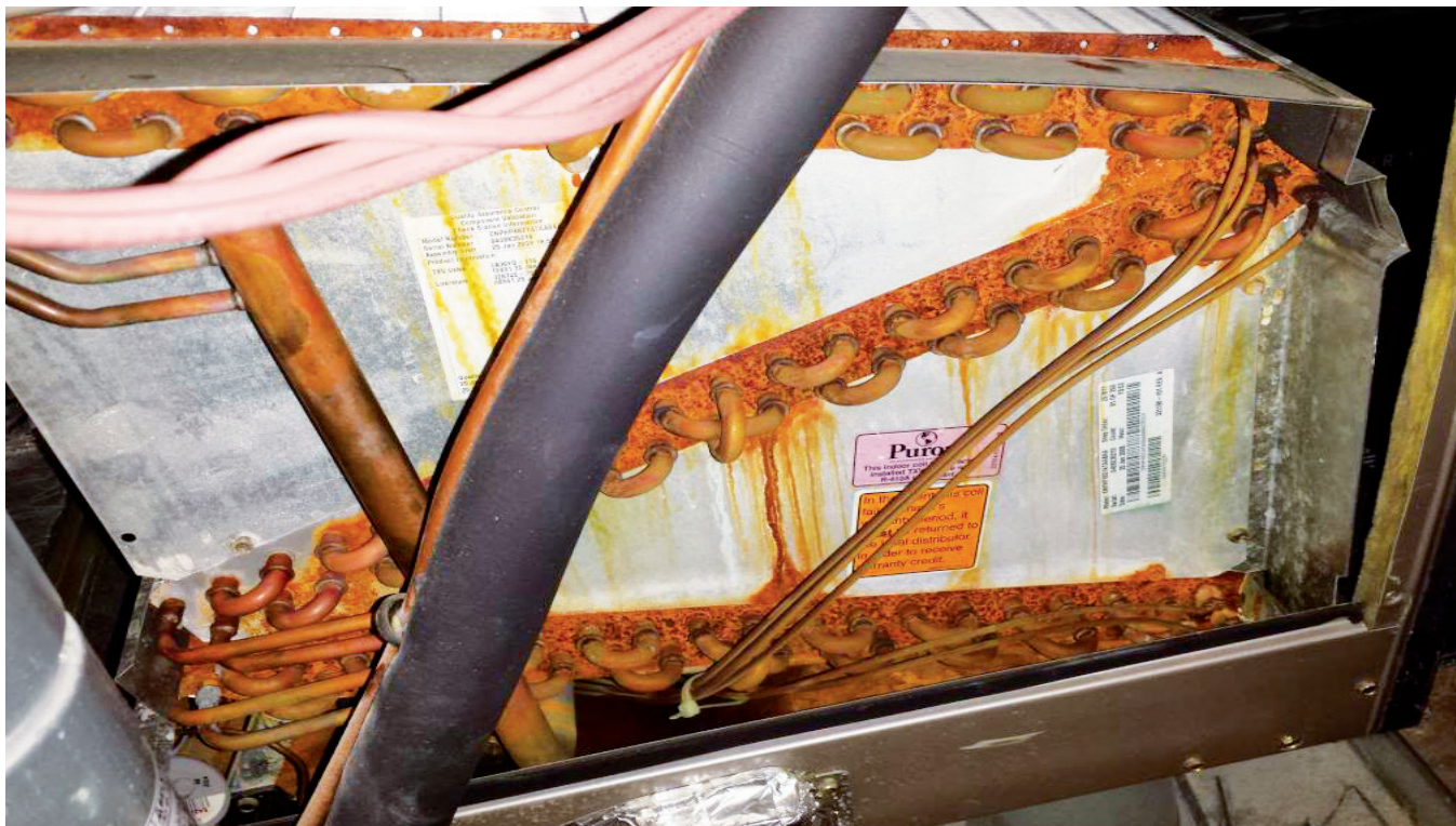
Formicary corrosion in a coil
