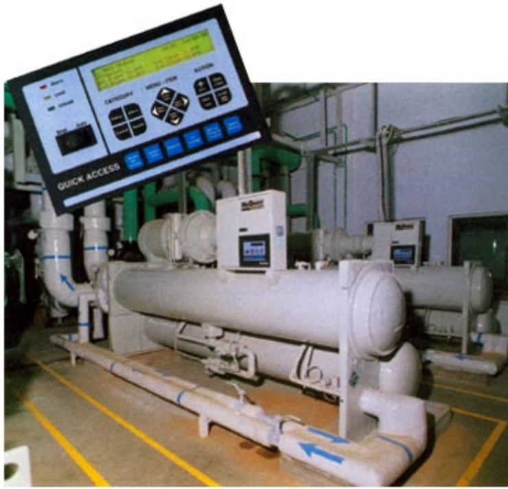
McQuay Centrifugal Chiller with Control Panel (Inset)
