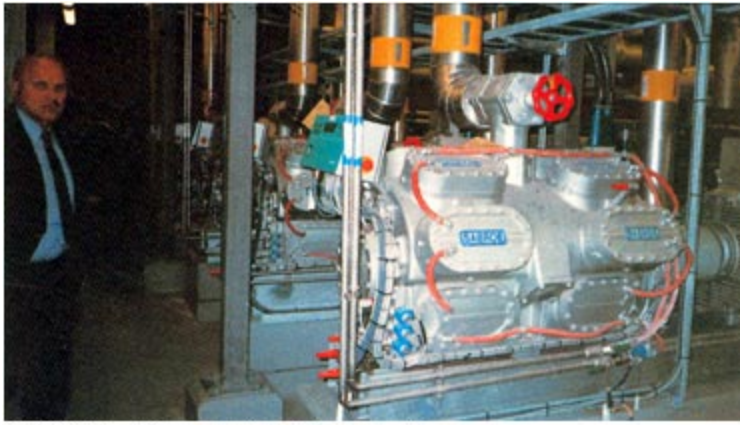
HVAC Plant Room at Oslo Airpoprt, Norway
