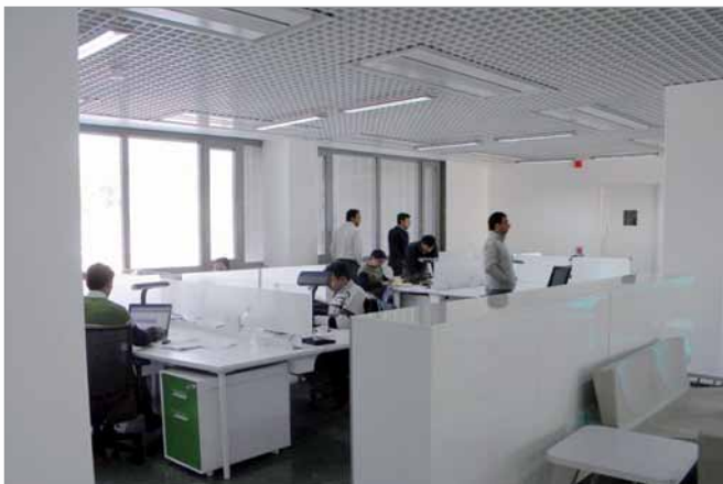
Photo 3: Chilled beam in the office space
