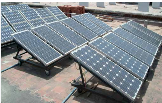
Photo 5: Solar PV on terrace
