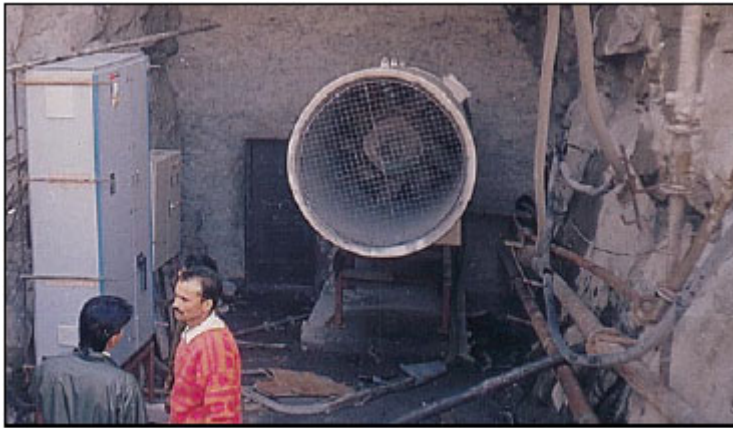
Tunnel ventilation fan with VFD at Chamera Hydel Power Project (H.P.)
