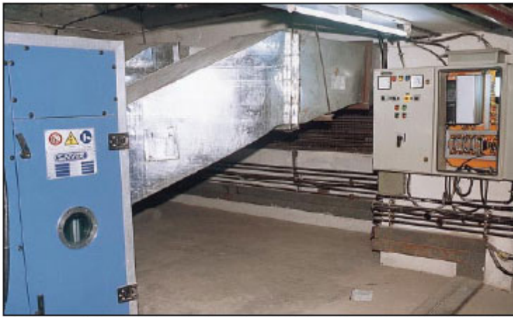
Air handling unit controlled by a VFD at the Taj Mahal Hotel, New Delhi
