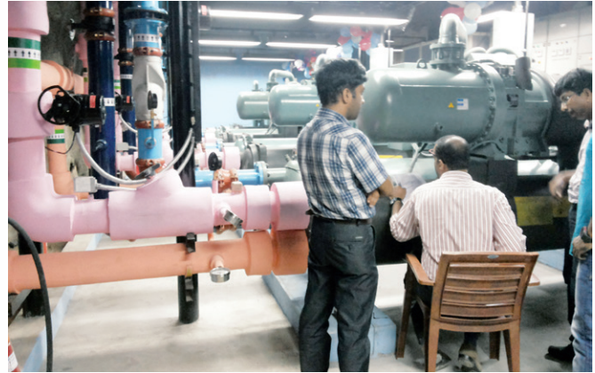
Photo 2: Grooved valves and fittings for chilled water and cooling water lines
