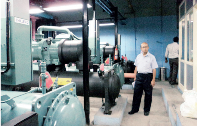
Photo 1: The author - facing the challenges in replacing a 34 year old underground plant
