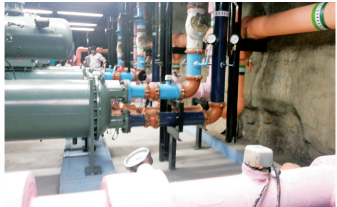
Photo 3: Grooved valves and fittings with tunnel rock in the background
