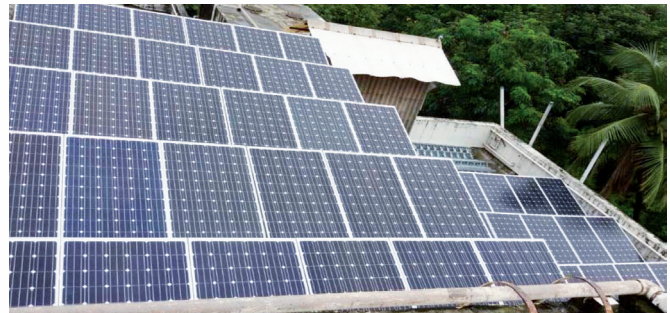
Photo 3: Off-site grid connected solar PV system
