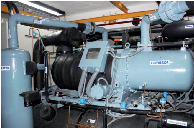
Photo 4: Energy efficient chiller installed at Bombay House
