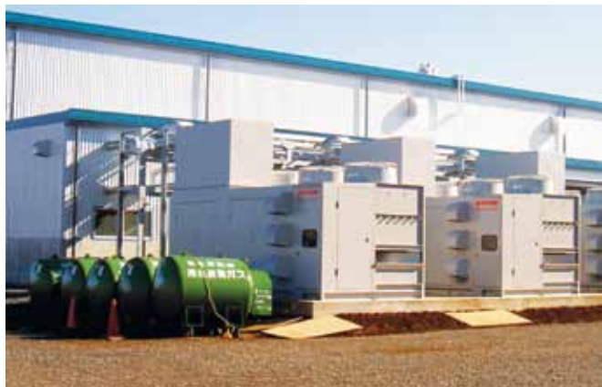
Photo 1 : CO 2 Indirect Package (Ice Plant)
