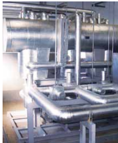
Photo 4 : CO 2 tank with CO 2 pump. Indoor Installation.
