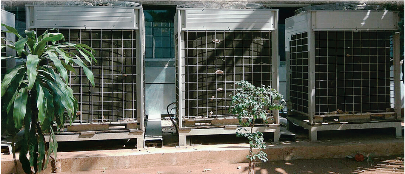
A VRF outdoor unit
