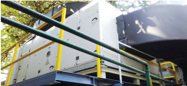
Photo 5: Thermal break air handling unit
