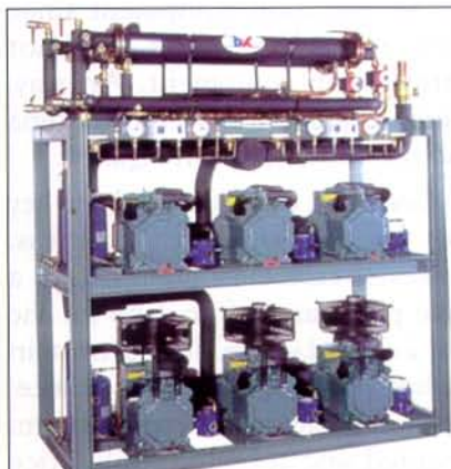
Figure 4: A low temperature rack with reciprocating compressors.
