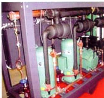
Figure 5: Two scrolls and one reciprocating compressor in parallel.
