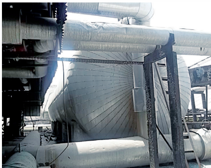
Crystal IT Park, Indore uses 3 x 2160 TR HR thermal storage tanks
