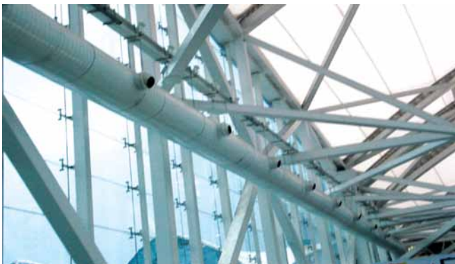
Supply air ducting with jet nozzles help with longer air throw at a reduced noise level
