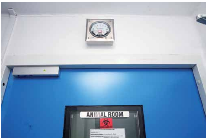
A magnahelic gauge indicating negative pressure inside the animal room
