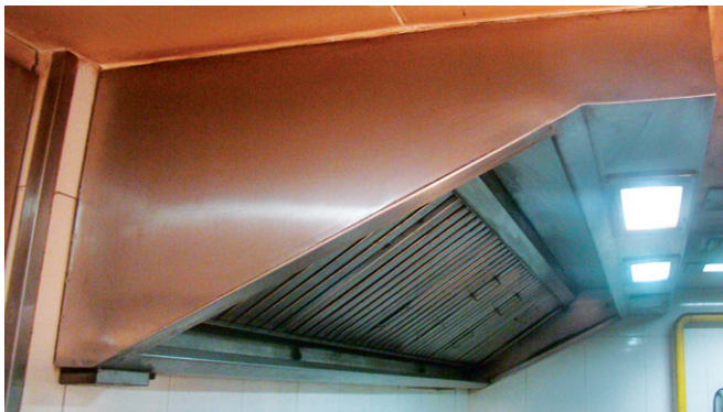
Photo 1: Wall mounted canopy hood
