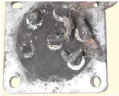
Figure 18 : Terminal box corroded.
