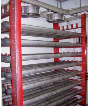
Photo 4 : One wall of a telecom shelter lined with PCM filled into aluminum pipes.
