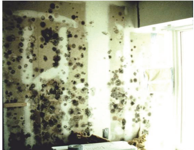
Photo 2: Heavy mould growth on a hotel wall
