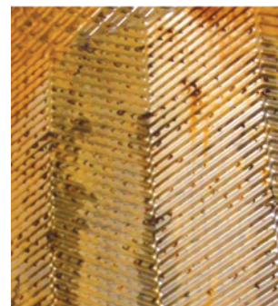
Figure 1. Fouling, not corrosion.
