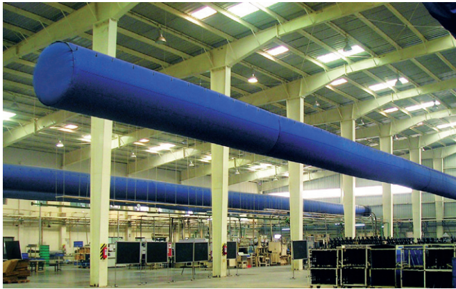
Figure 3: A fabric duct in the Tenneco India plant at Bawal, Haryana
