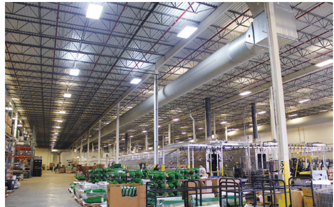
Figure 2: Fabric duct in the paint area of a factory
