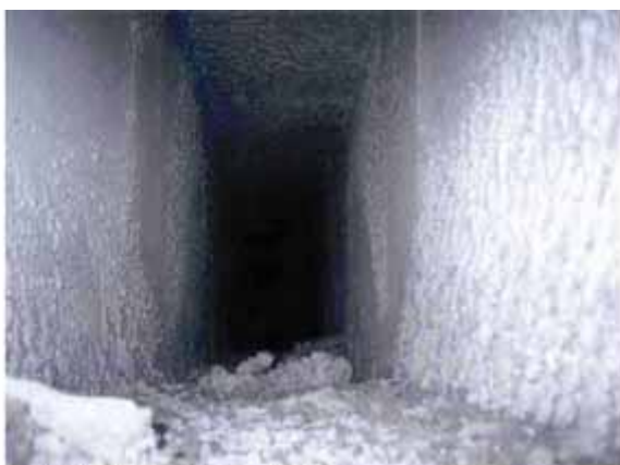
Air distribution duct before cleaning.
