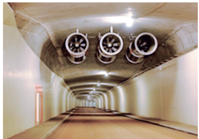
Figure 7: Tunnel fans for exit-entry points of underground car park
