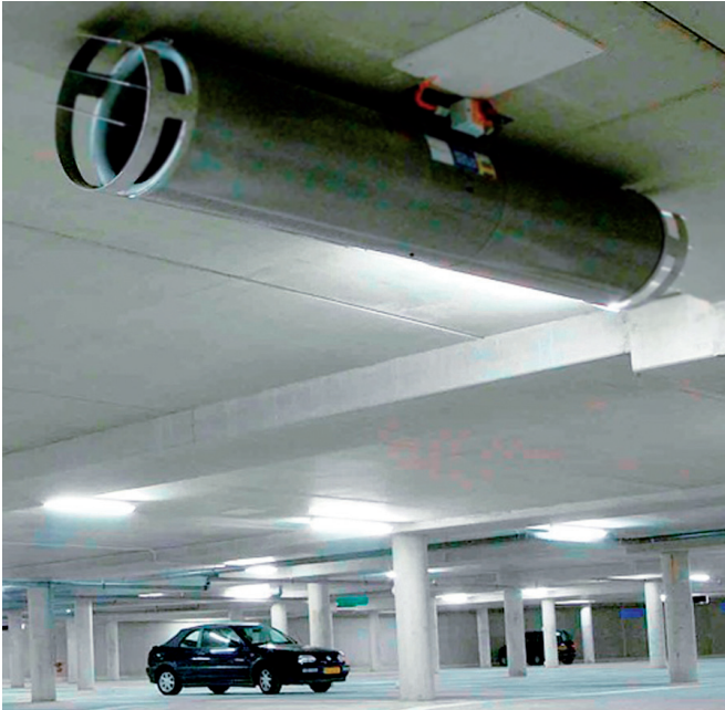
Figure 2: Jet fan used for car park ventilation
