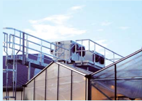
Split refrigeration system
