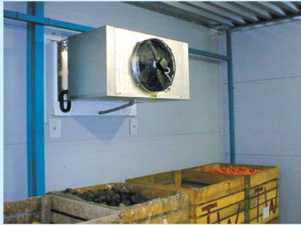
Uniblock refrigeration system
