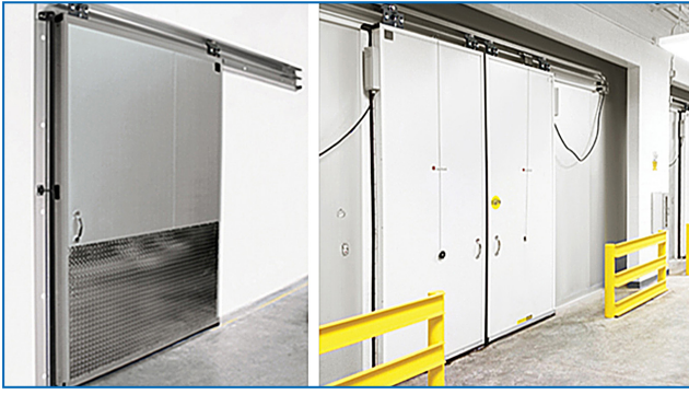
Figure 5-13: Horizontal sliding doors with safety guard
