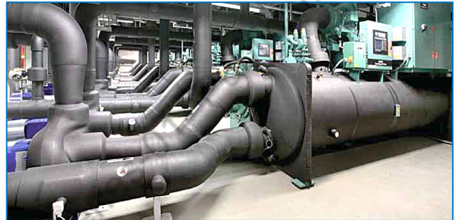
Figure 6-23: Chiller insulation with piping
