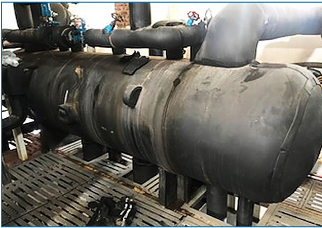
Figure 6-20: Insulated L.P. vessel in operation for last ten years
