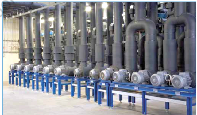
Figure 6-24: Chilled water distribution insulation
