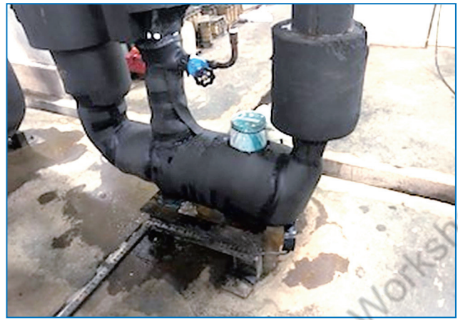
Figure 6-22: Liquid ammonia pump insulation
