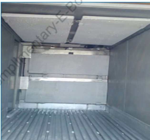
Figure 8-7: Ceiling mounted eutectic plates
