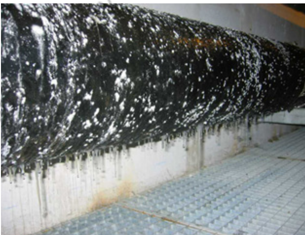
Figure 4-2: Condensation on pipe
