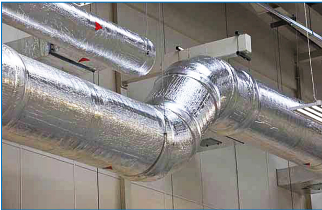
Figure 6-27: Insulation protected by aluminium foil lamination vapour barrier
