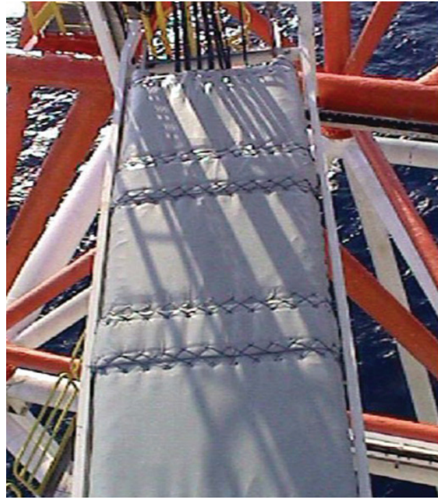
Figure 7-18: Cable Trays Insulation
