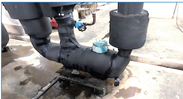
Figure 6-26: Liquid ammonia pump insulation
