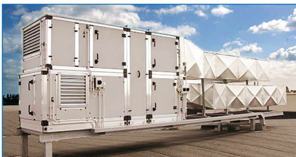
Figure 7-7: AHU installed out
