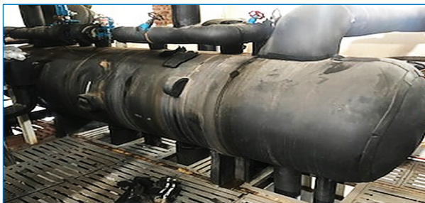
Figure 6-24: Insulated L.P. vessel
