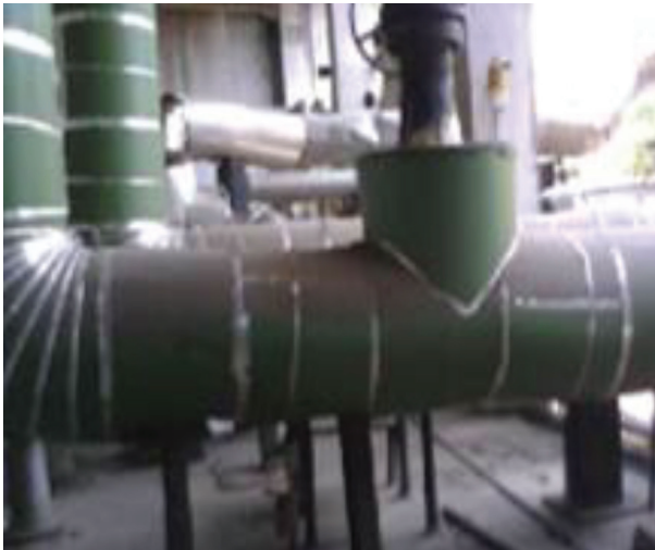
Figure 6-7: PPGI Sheet Cladding
