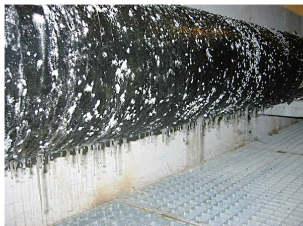
Figure 4-2: Condensation on pipe
