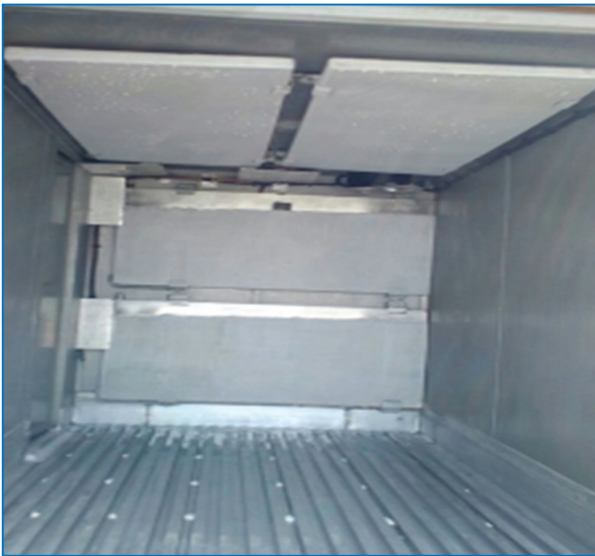
Figure 8-7: Ceiling mounted eutectic plates
