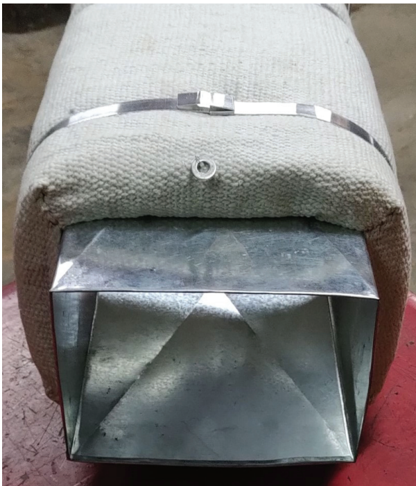
Figure 7-12: Encased Insulation over GI Duct
