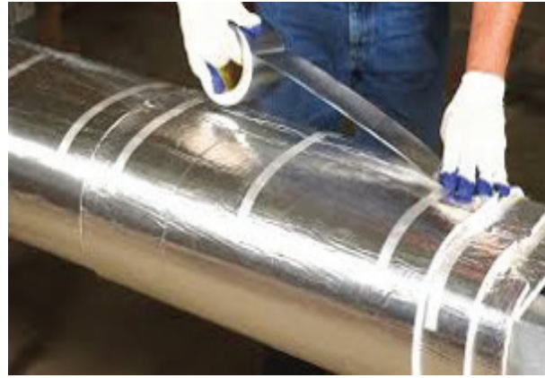
Figure 7-13: Encased Insulation joints sealed with tape
