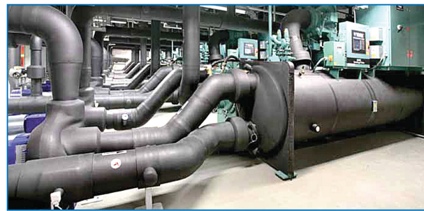
Figure 6-27: Chiller insulation with piping
