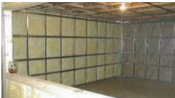
Figure 13.11: Plant/AHU room acoustic lining
