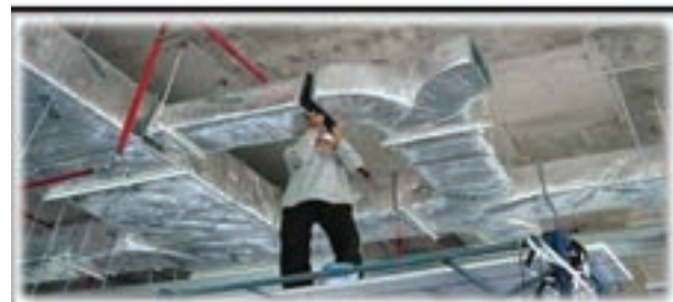
Figure 13.7 a, b: Duct insulation with Rockwool/glass wool
