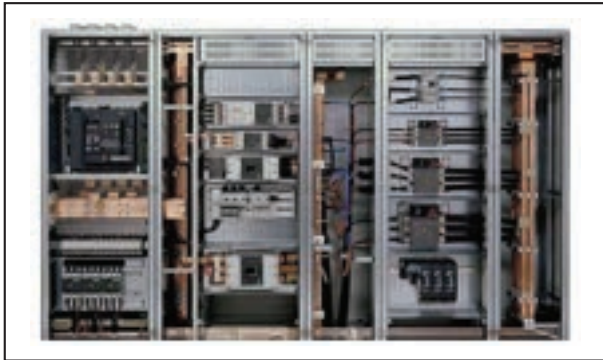
Figure 17.2: Open view of electrical panel
