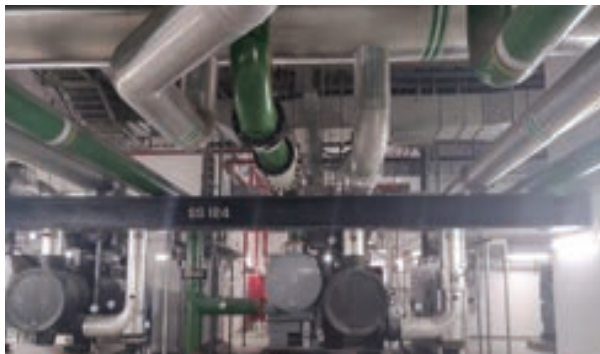
Figure 1.2: Chiller plant room
