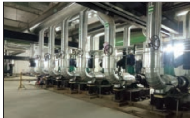
Figure 13.6: Piping with insulation finished with aluminum cladding
