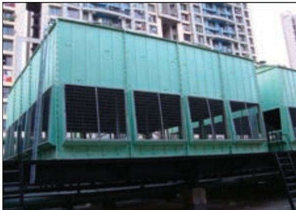
Figure 6.8: Large cooling tower located close to residential building (not acceptable)
