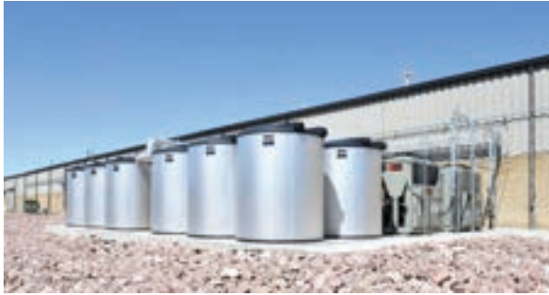
Figure 15.1 (b): Ice based thermal storage tanks
