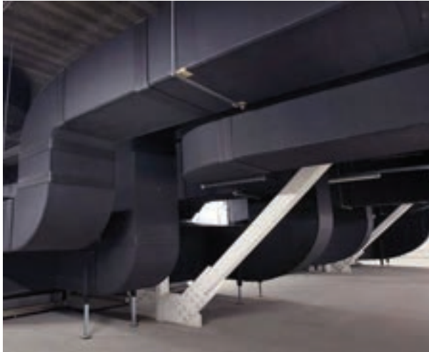
Figure 13.8: Duct insulation with nitrile rubber
