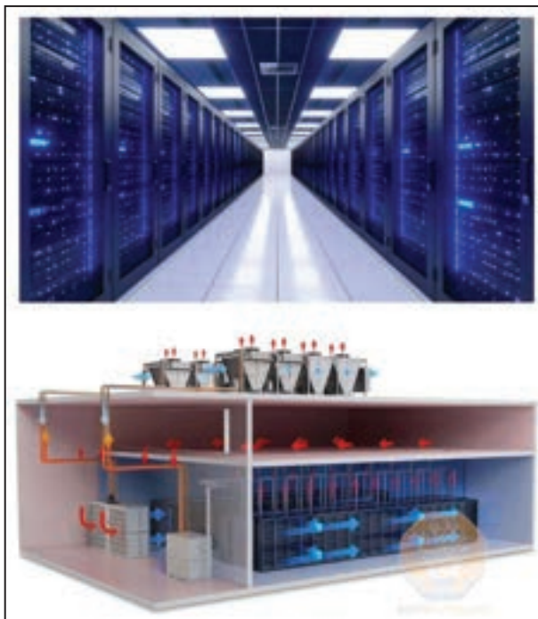
Figure 16.9: Data centers and typical cooling arrangement
