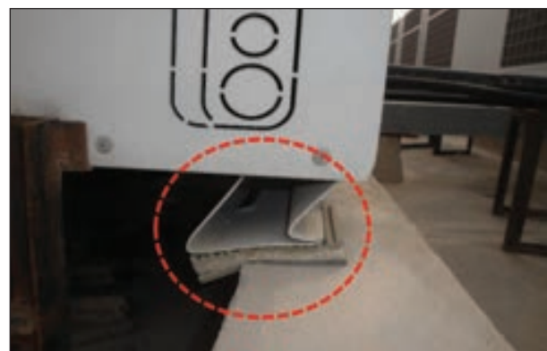
Figure 4.5: Outdoor unit installation – wrong practice
