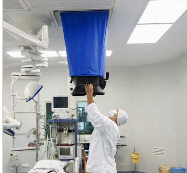
Figure 8: Airflow Measurement with Capture Hood
